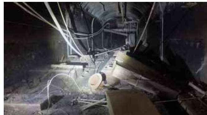
Battery Arizona Power Room
