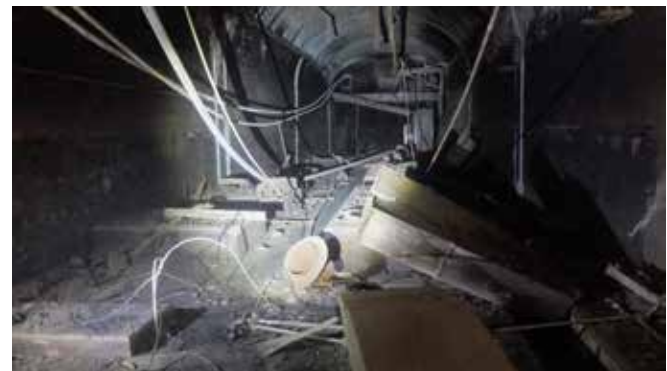
Battery Arizona Power Room
