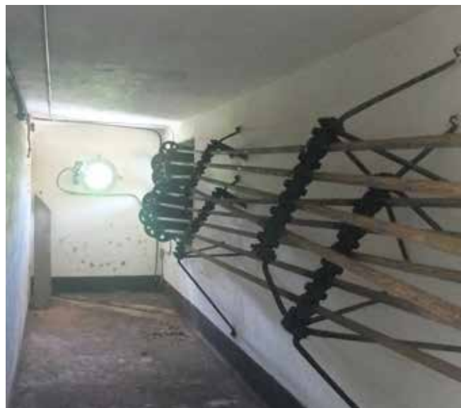
Intact mechanical indicator display mechanism at Battery Harlow
