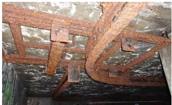
Fort Dearborn Battery Seaman overhead trolley system
