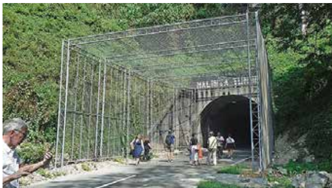
Protective barriers against rock slides at West Entrance
