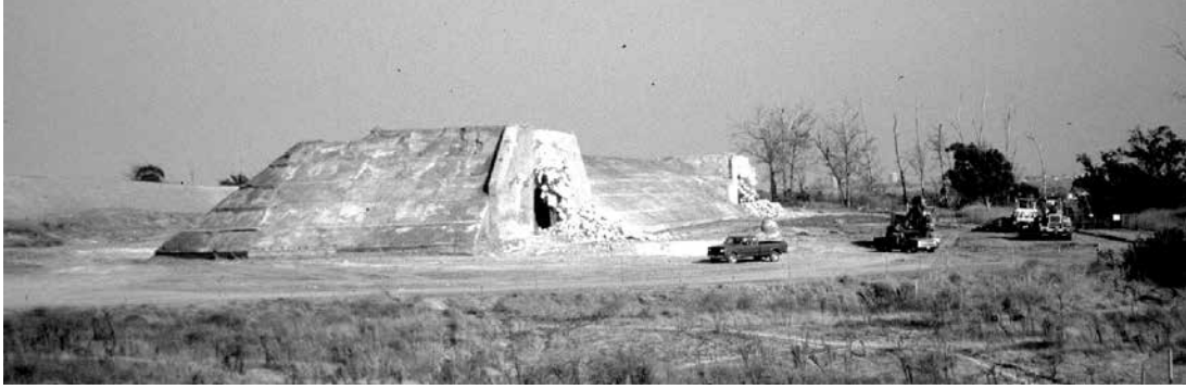
BCN 128, Bolsa Chica, being demolished 1993 (photo by Mark Berhow). The Bolsa Chica site is now mostly in private hands, the battery structures were destroyed 1993-1995 for a housing development. A section with the Panama mounts is part of a marine preserve.
