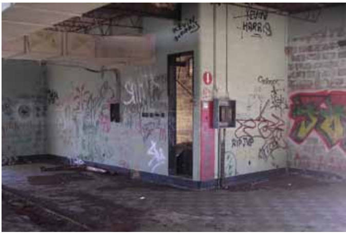
Generator Building interior
